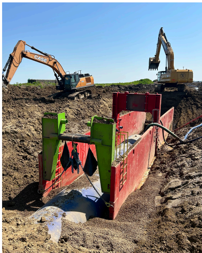
Red River Valley Water Supply Project 72-inch pipeline installation near Carrington, ND.
